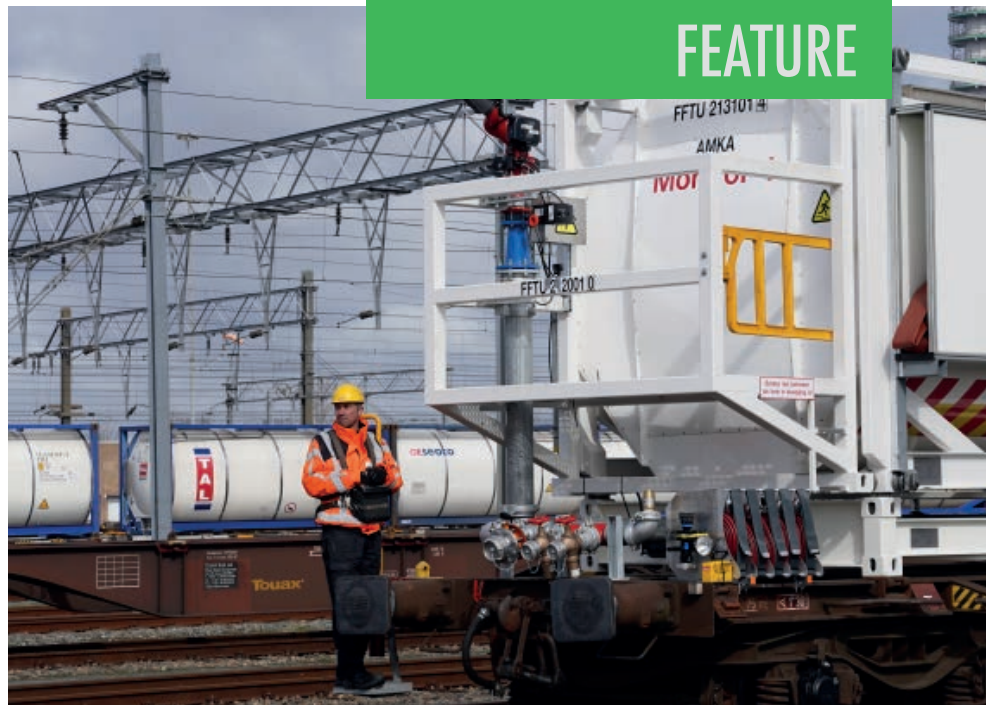
Remote controlled 4,000 L/min monitors are mounted on platforms at both ends of the train, handlines can be attached for manual foam application
